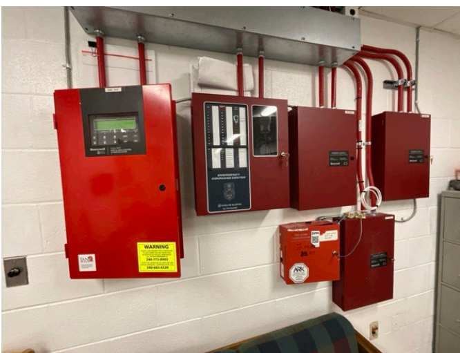
23 - FIRE ALARM PANEL
