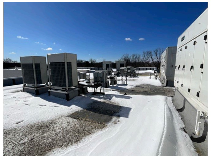
28 - ROOF TOP HVAC
